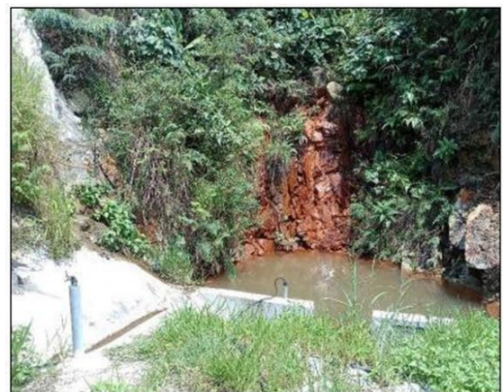
Figure 2. Continuous water seepage through fractured igneous rock
