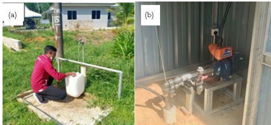
Figure 1: Groundwater sample collection from (a) faucet connected to the (b) pump of the tube well.
